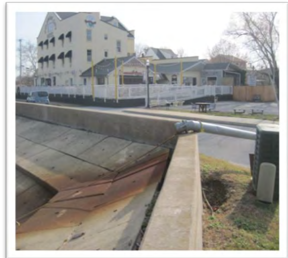
Figure 5-4. Pump outfall at Stauffer Slip, at the end of Washington Street.
